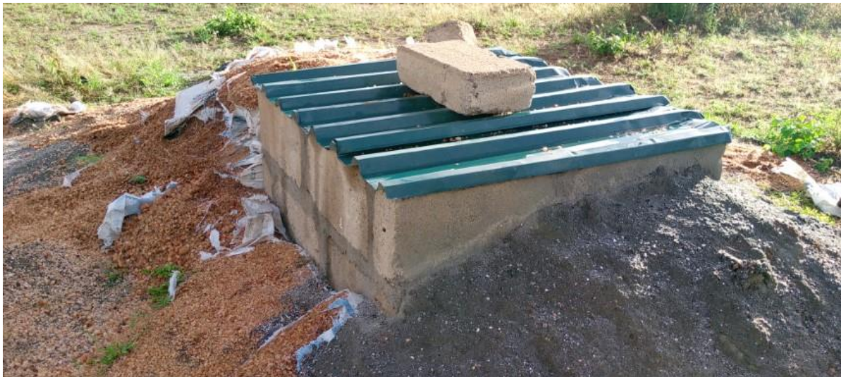
A borehole station chamber covered to protect the installed pump and motor machine to support water from the borehole remain sustainable at the project center.
